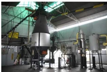
Rice Husk based 250 kWe Power Plant, India
