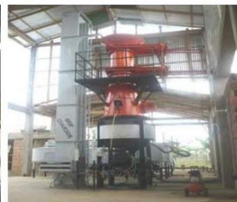
40 kWe Power Plant, Colombia
